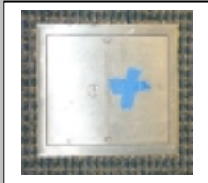
Floor box to Data ports
